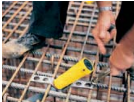
Anchor system is easily fixed to the reinforcement with wire and pliers.
