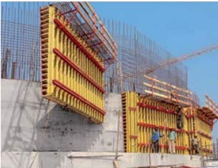
VARIO VT 20 being used to construct a circular tank. Timber on top of VT girders and steel walers produce the circular shape.
