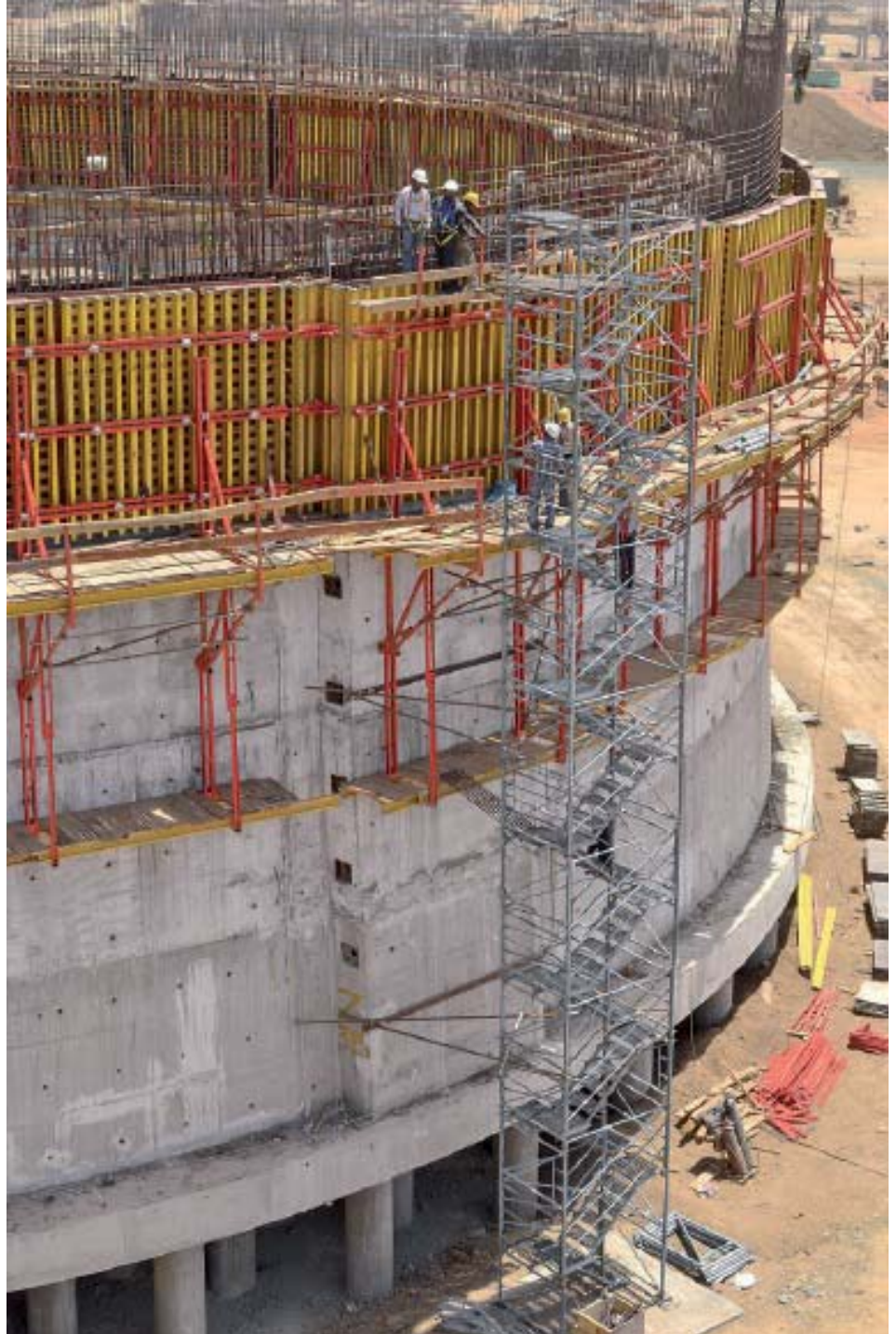
Silo, h = 20 m, Ø = 47 m for 3 storage tank for ethylene, India. Shuttered with circular VARIO VT20 girder formwork on CB 240 climbing system.
